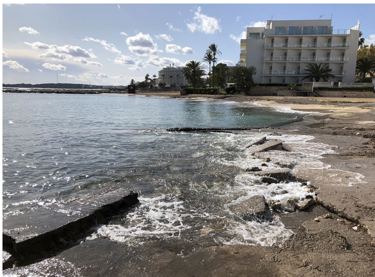
Figure 5. Concrete blocks used to prevent the erosion of Cala Bona beach
